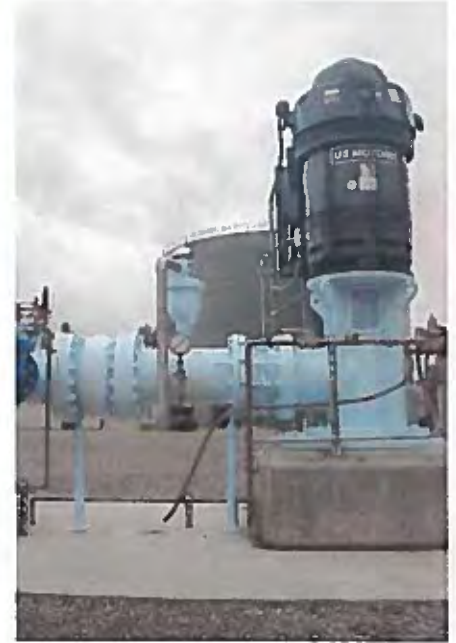
Rockwood Water PUD Groundwater System
