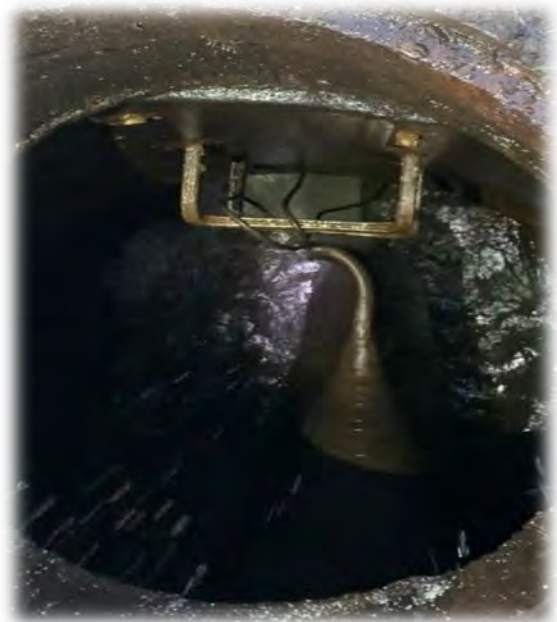
4) Plant bypass manhole #2 duckbill
