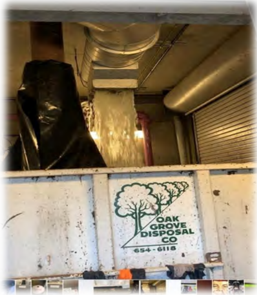
1) Flooding in headworks
