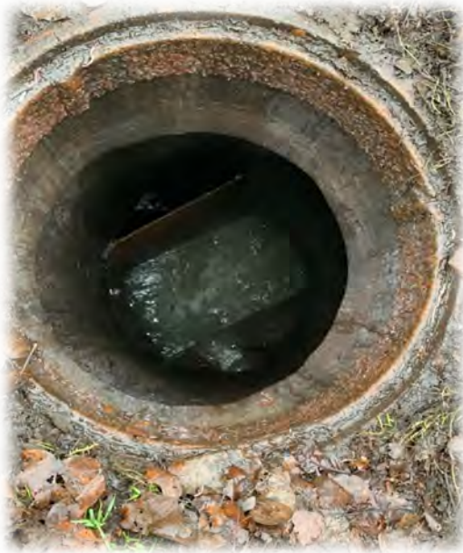
3) Plant bypass manhole weir
