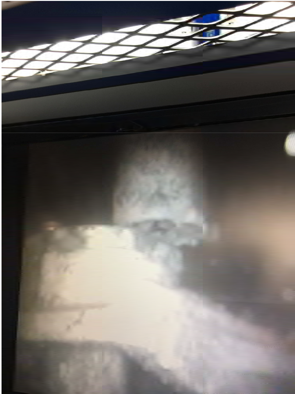
Photo 1 Underwater shot of broken shaft operating UV gate #2
