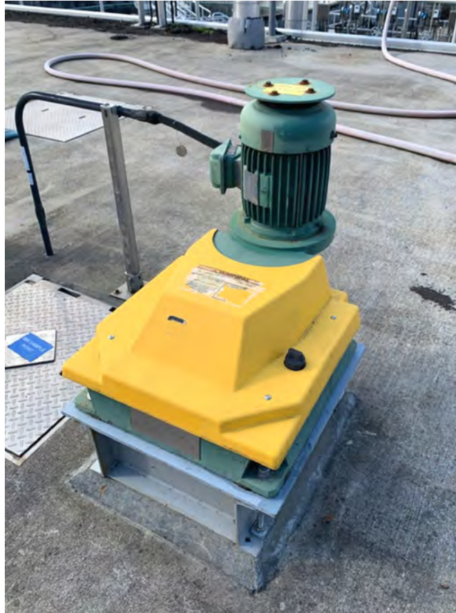
Figure 38. Aerobic Digesters 1 and 2 vertical turbine mixer motor
