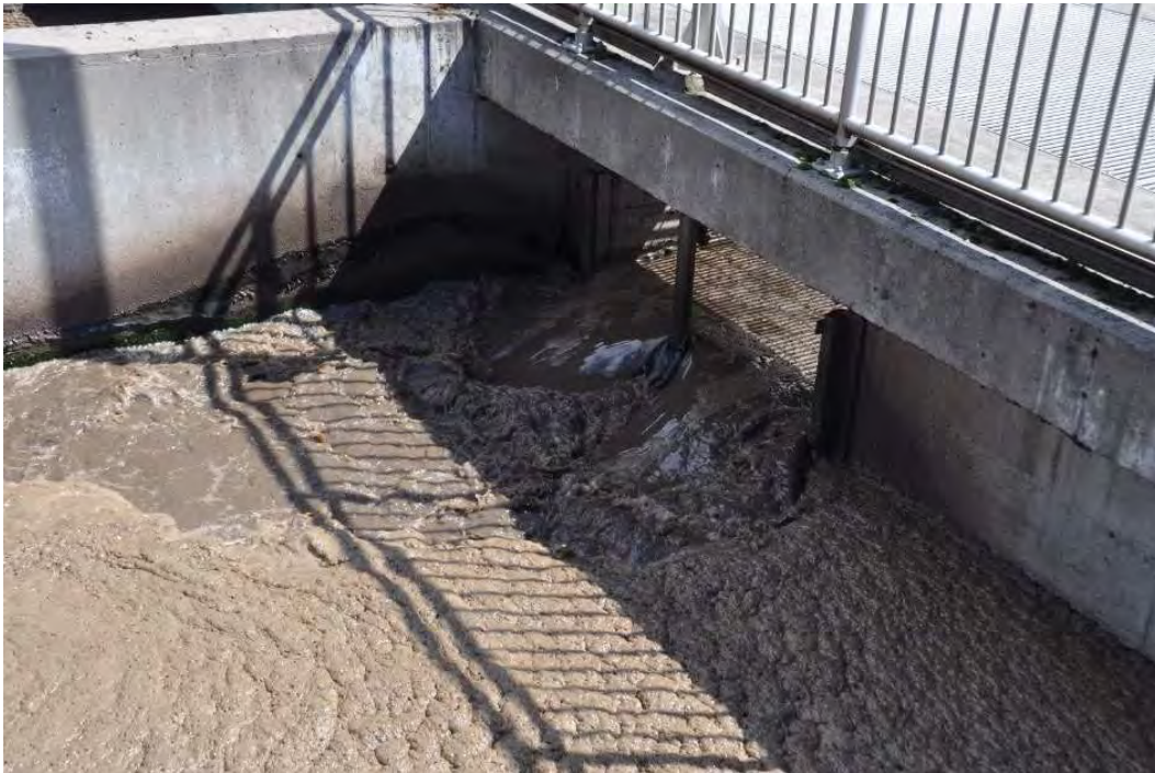
Figure 18. Hydraulic restriction at aeration basin weir gate
