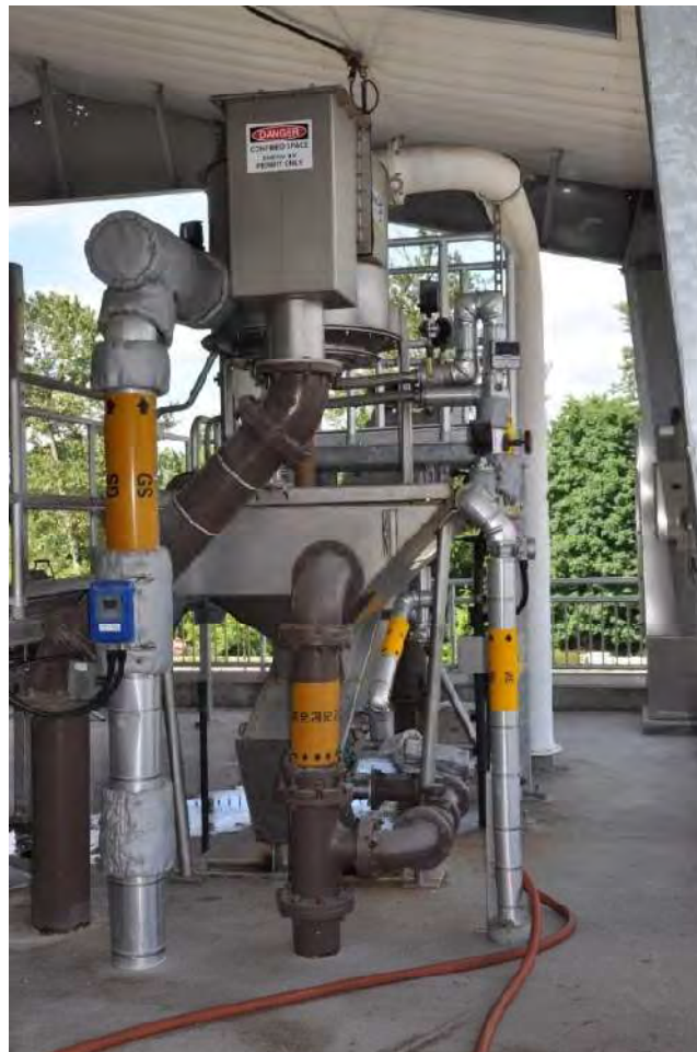
Figure 19. Grit washing and dewatering equipment
