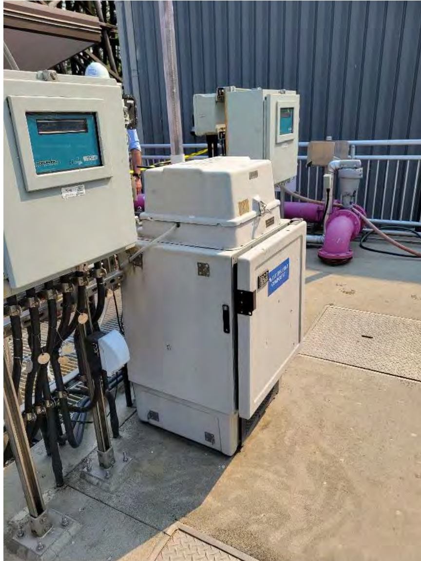
Figure 35. Effluent flow meter panels and composite sampler
