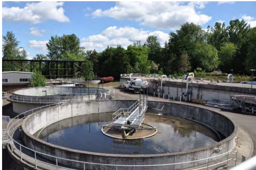
Figure 23. Newer secondary clarifier
