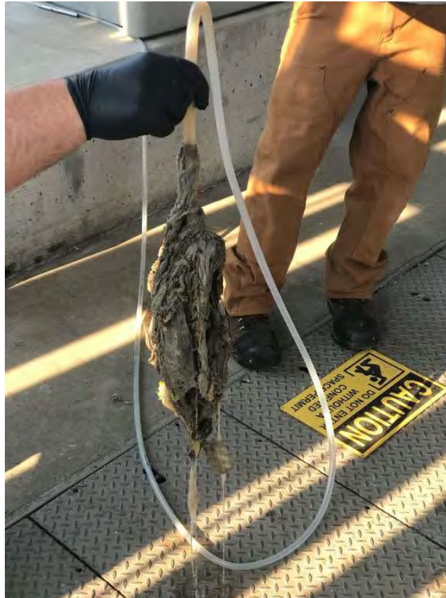
Figure 9. Debris accumulation on influent sampler suction strainer
