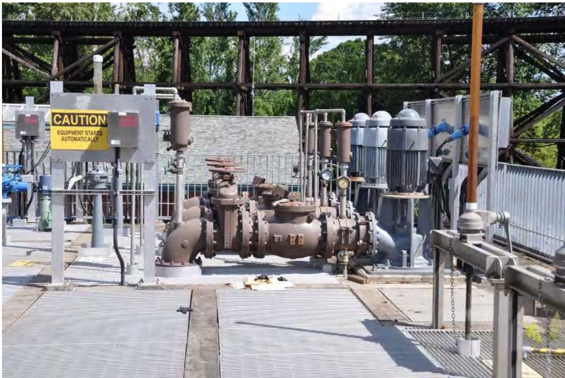
Figure 25. Internal mixed liquor recycle pumps
