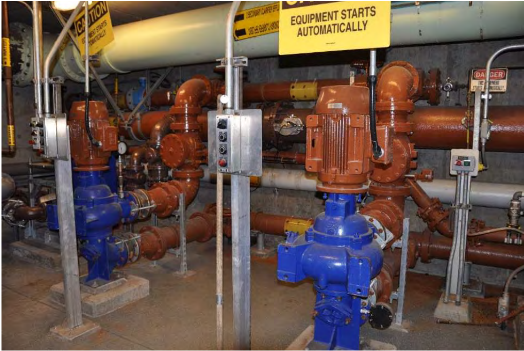
Figure 27. IBR feed pumps in RAS/WAS pump station
