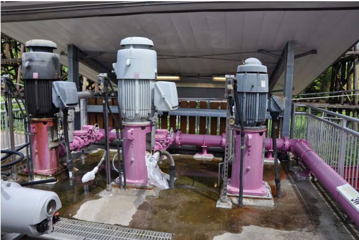
Figure 34. 3W pumps located at the disinfection facility
