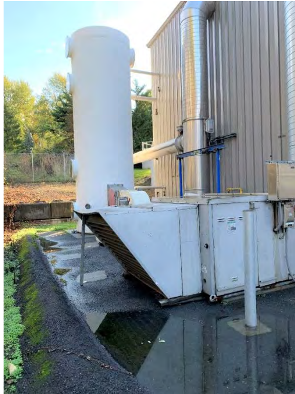
Figure 53. Chemical scrubber tower and foul air fan
