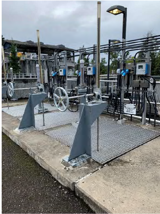
Figure 32. East RAS pumps
