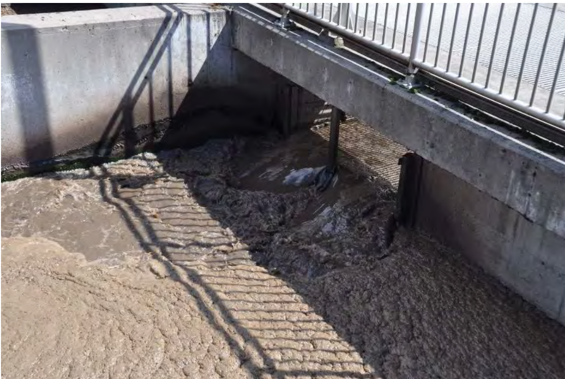
Figure 23. Hydraulic restriction trapping foam at aeration basin horseshoe turn
