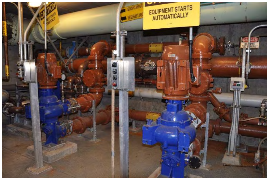
Figure 21. IBR feed pump in RAS/WAS Pump Station
