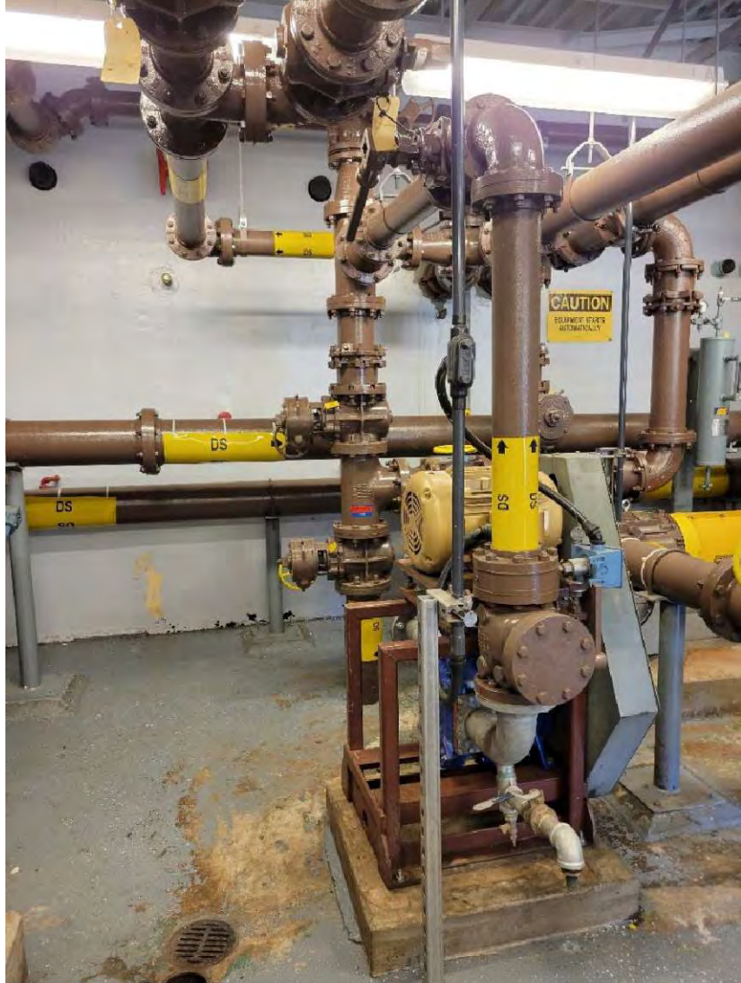
Figure 31. Digested sludge pump
