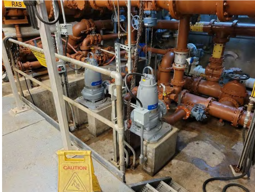
Figure 24. RAS pumps in RAS/WAS Pump Station
