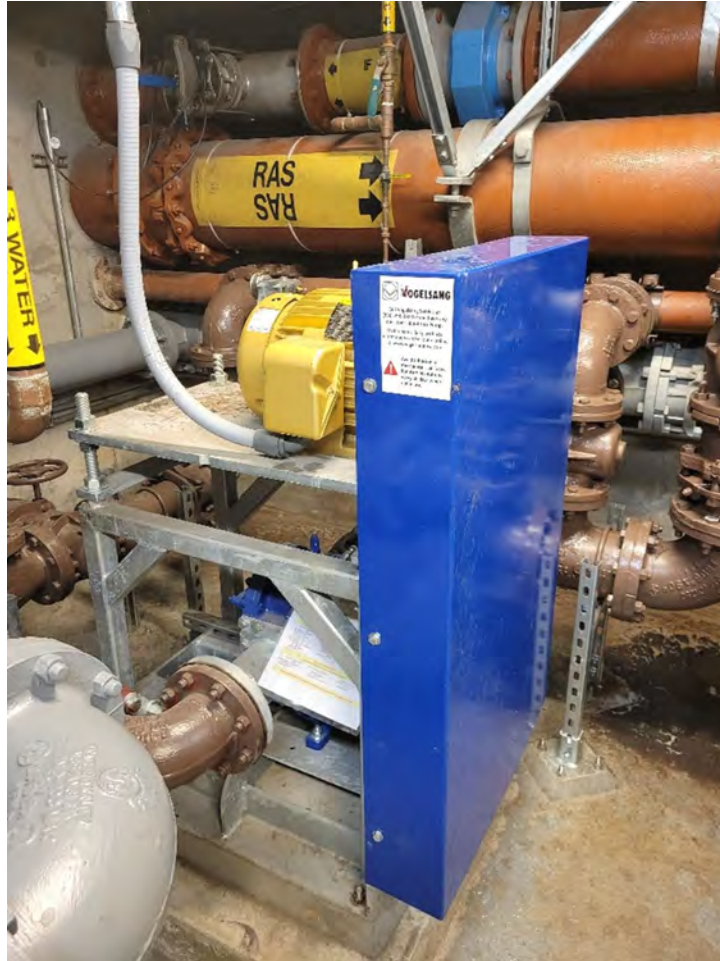
Figure 28. WAS Pump 3 in RAS/WAS pump station
