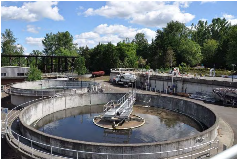
Figure 30. Newer secondary clarifier
