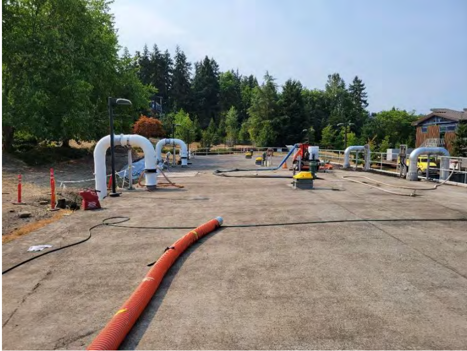
Figure 36. Top of Aerobic Digesters 1 and 2
