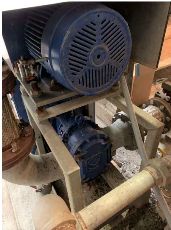
Figure 44. Thickened waste activated sludge pump
