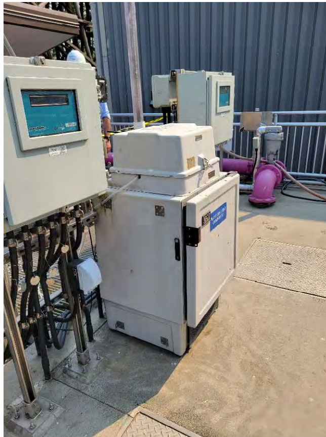
Figure 27. Effluent flow meter panels and composite sampler
