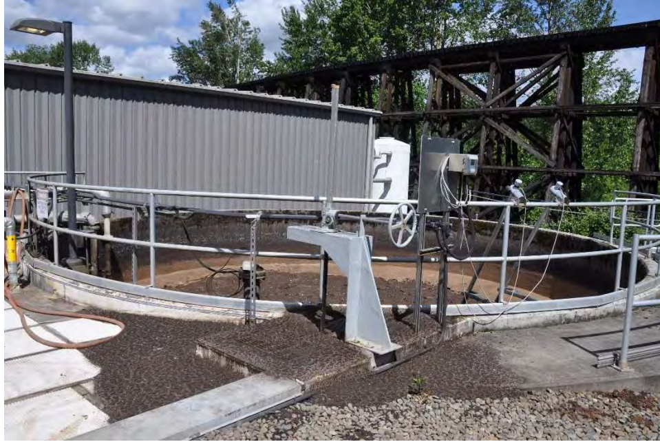
Figure 39. Circular aerobic digester
