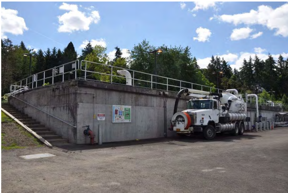
Figure 37. Aerobic Digesters 1 and 2 from below
