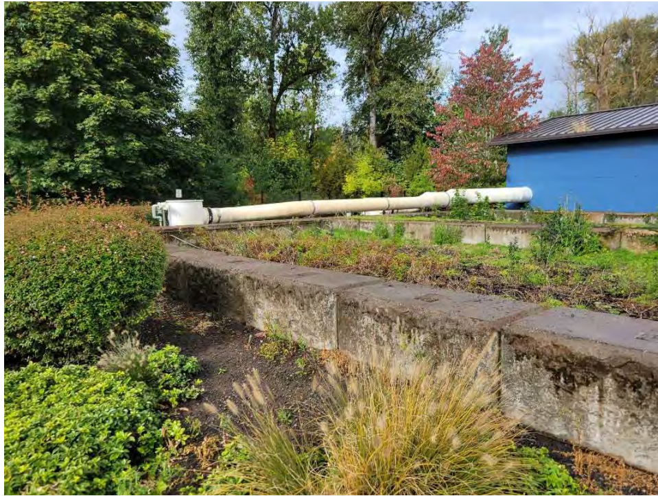
Figure 52. Biofilter building and foul air piping
