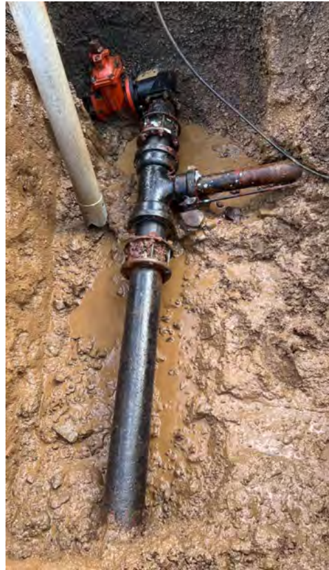
Lead tee with 4" hydrant
