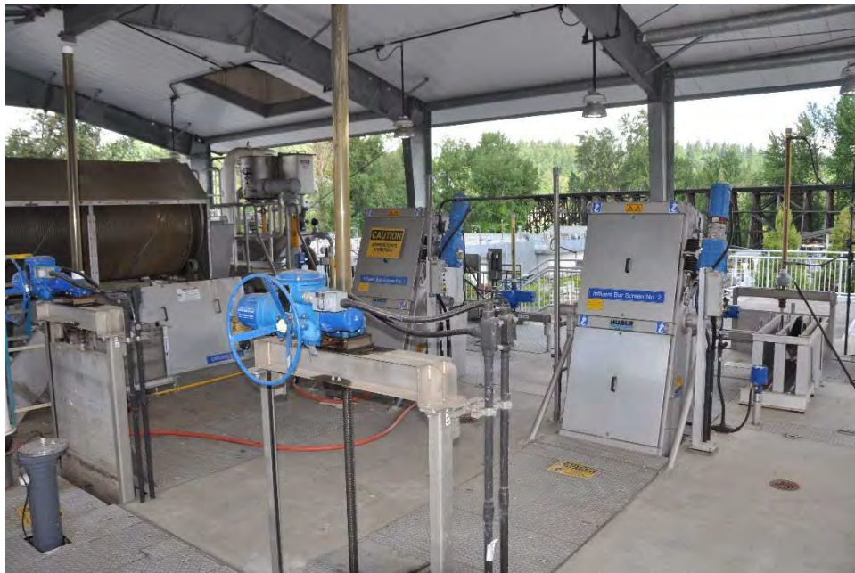
Figure 12. Influent screens with influent and effluent gates
