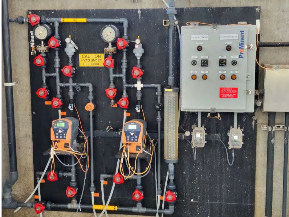
Figure 48. Sodium hypochlorite metering system
