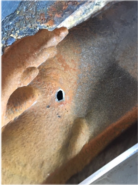
Hole in Digester Pump #2 plate
