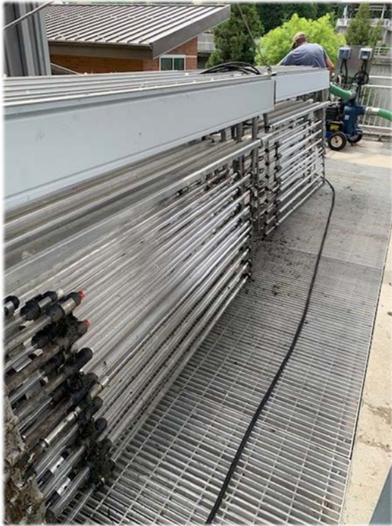
UV Bulb Racks removed for cleaning
