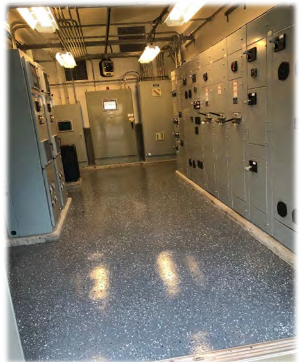
Building 75 Motor Control Center
