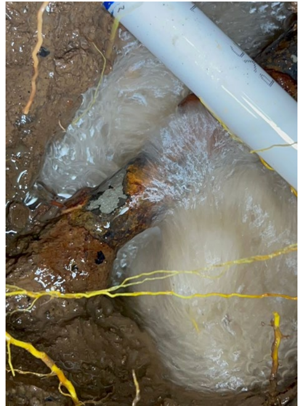
Photo 6: Leaking service on Orchard Lane
