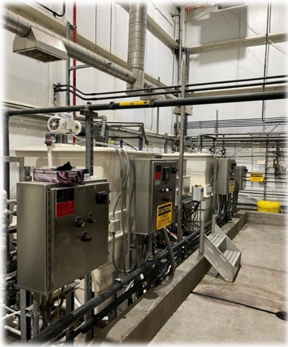
Older dry polymer system.
