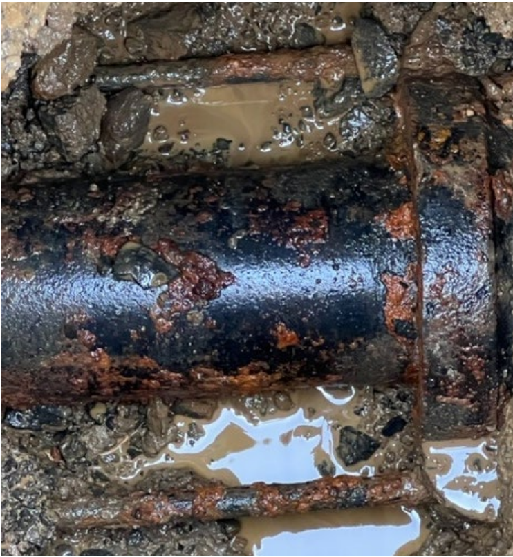
Photo 5: Slow leak found on fire hydrant lateral
