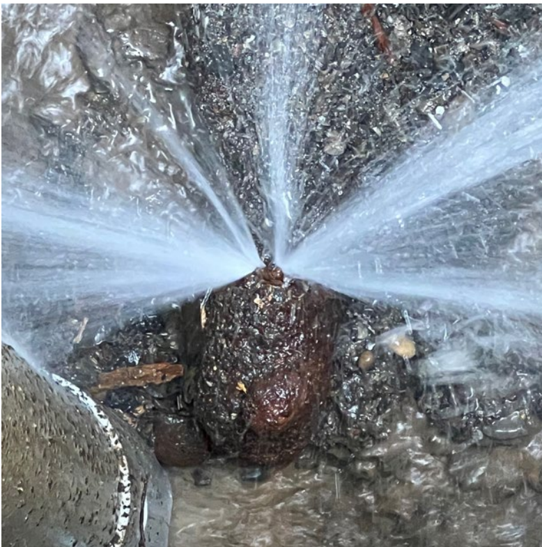
Photo 7: Leaking 2-inch galvanized pipe on 28 th Ave.
