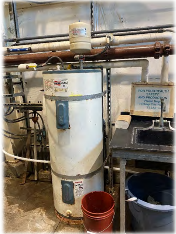
Old Hot Water Heater
