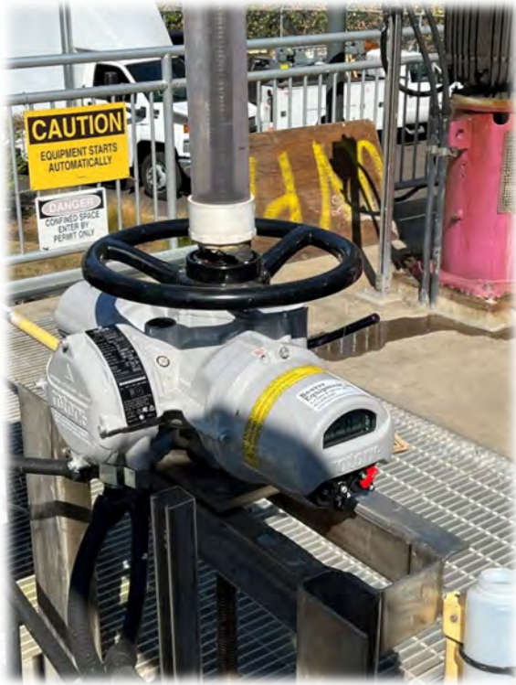
New Weir Gate Actuator
