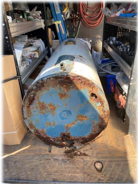
Old Hot Water Heater Rusted Out
