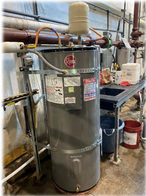
New Hot Water Heater Installed
