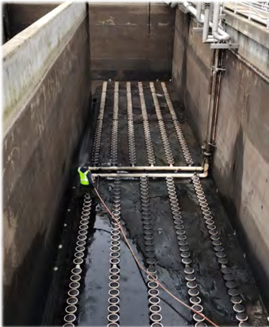
Aeration Basin #3 cleaning Randy Leniger hosing
