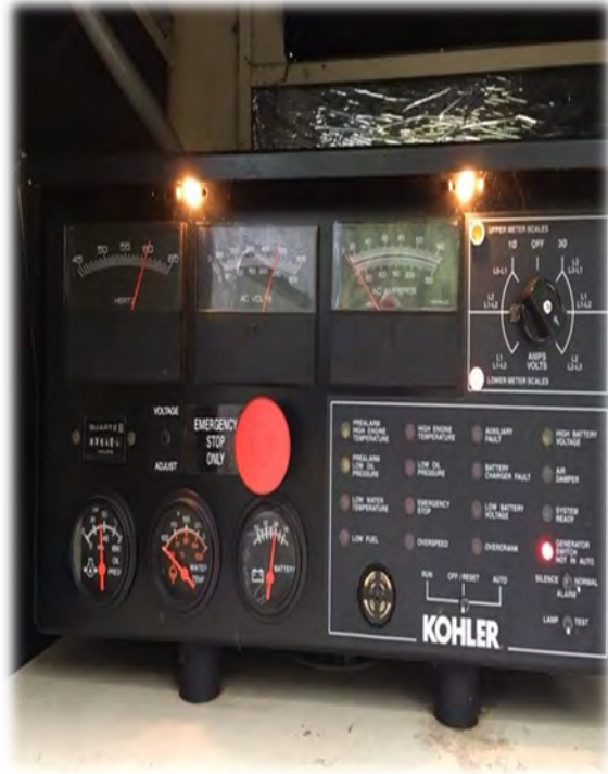
2. Engine generator running with no problems.
