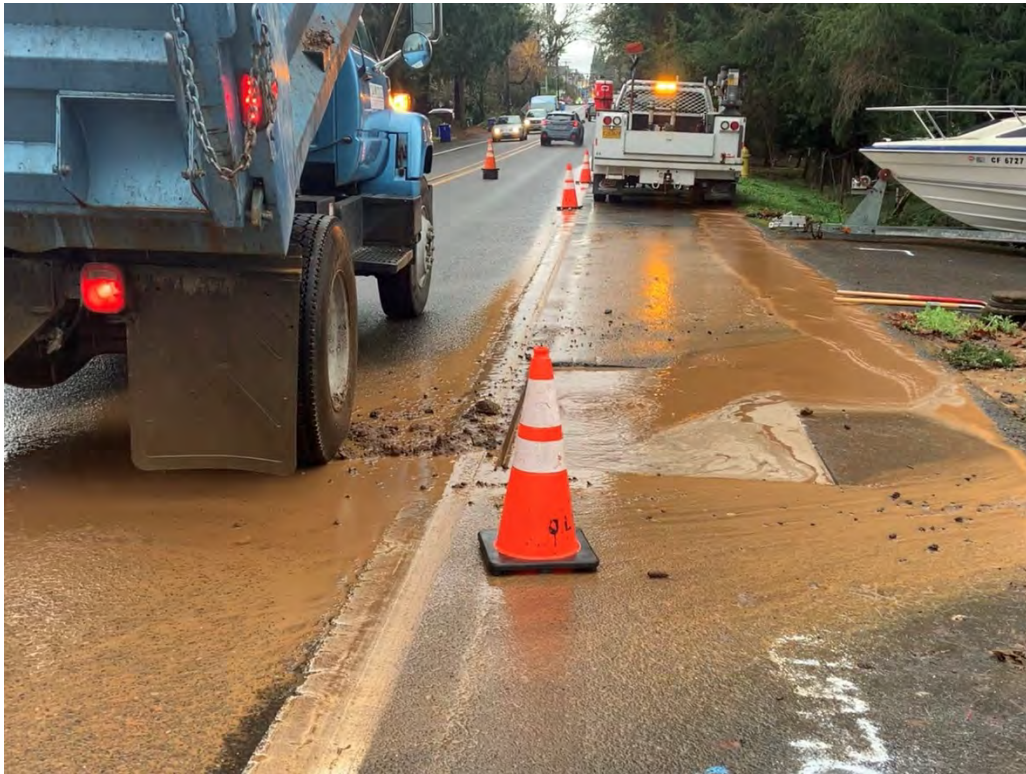
Photo 8: Main leak on River Rd.
