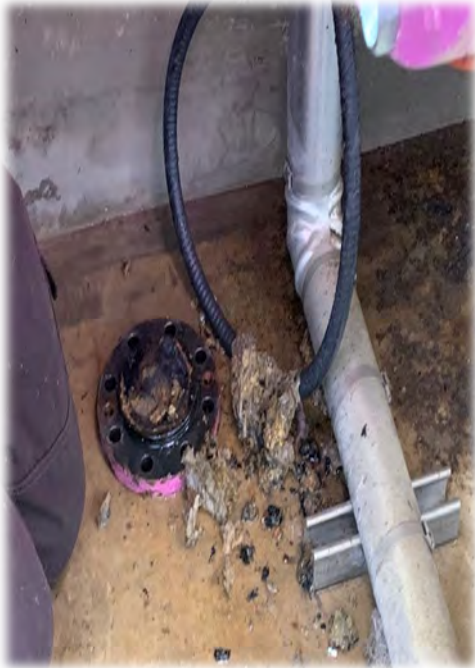
Gunk from heavy flows clogged the reuse strainer.
