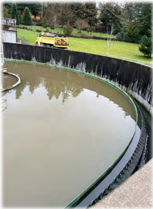
Upset Clarifier the week of January 17.
