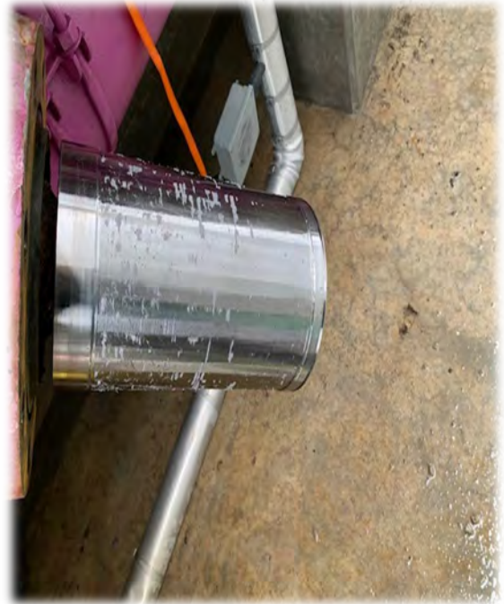
Strainer clean and ready to go back online.
