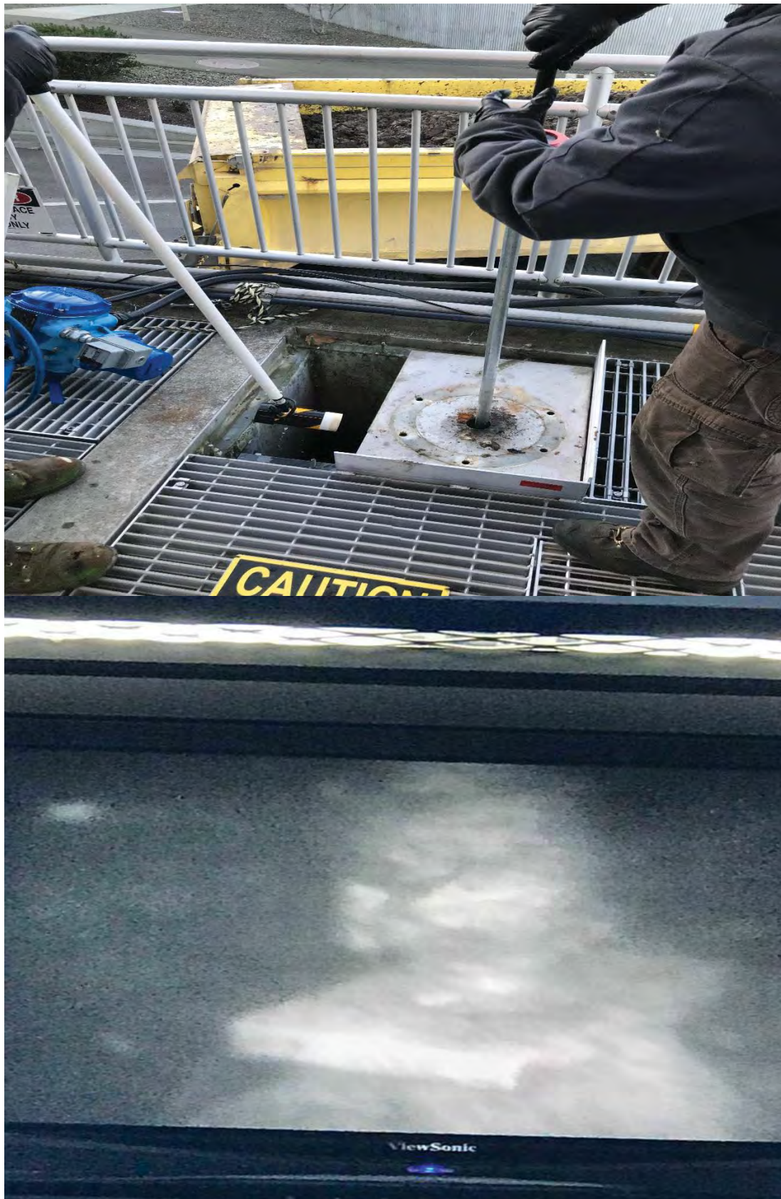
Photo 7&8 Camera use Shot is 20 ft underwater of the connection point (looked better on the screen)
