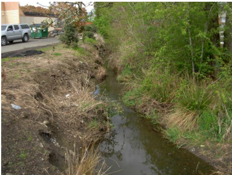
Site location: 015 Photo number: 044 Description: Incised channel and active eroding stream banks
