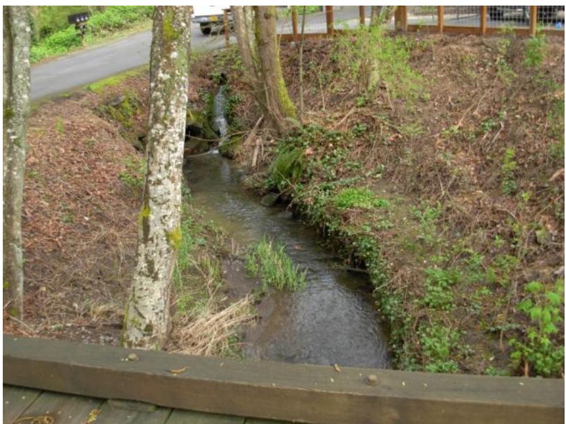
Site location: 006 Photo number: 002 Description: Public ROW - Downstream of bridge at Fair Oaks Ave.
