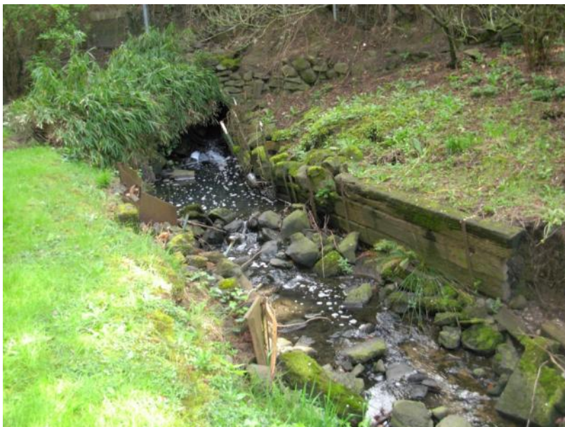
Site location: 012 Photo number: 032 Description: Private Property (3320 West View Ave). Reflects limited daylighted channel in backyard.
