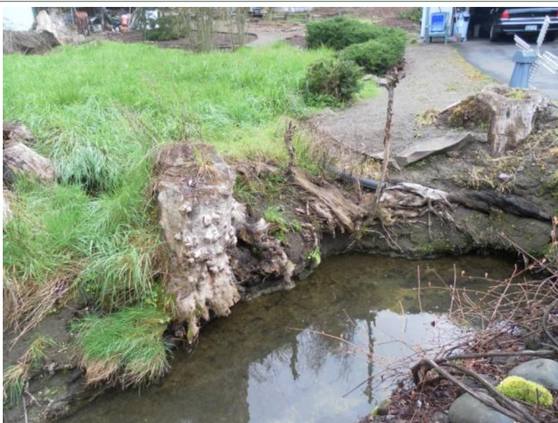
Site location: 002 Photo number: SAM_1202 Description: Private Property (15320 SE Laurie Ave). Exposed roots on eroding bank
