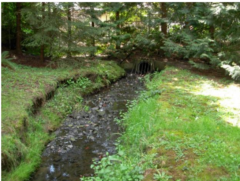
Site location: 013 Photo number: 036 Description: Looking downstream to culvert under adjacent manufactured home park.
