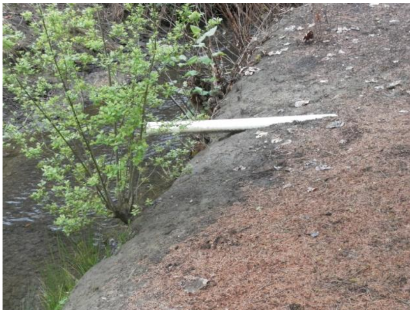
Site location: 002 Photo number: SAM_1209 Description: Private Property (15320 SE Laurie Ave). Area drain showing extent of channel widening (1 foot+ over 1 year)
