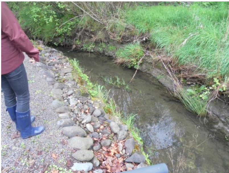
Site location: 002 Photo number: SAM_1201 Description: Private Property (15320 SE Laurie Ave). Channel reinforcement on inner bank.
