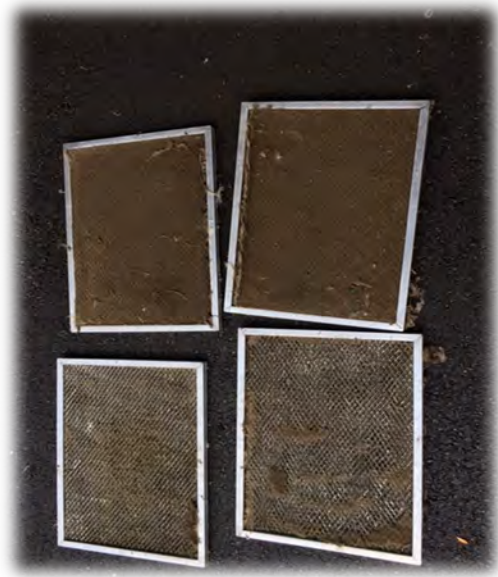
2) Air Handling pre-filters post smoke
