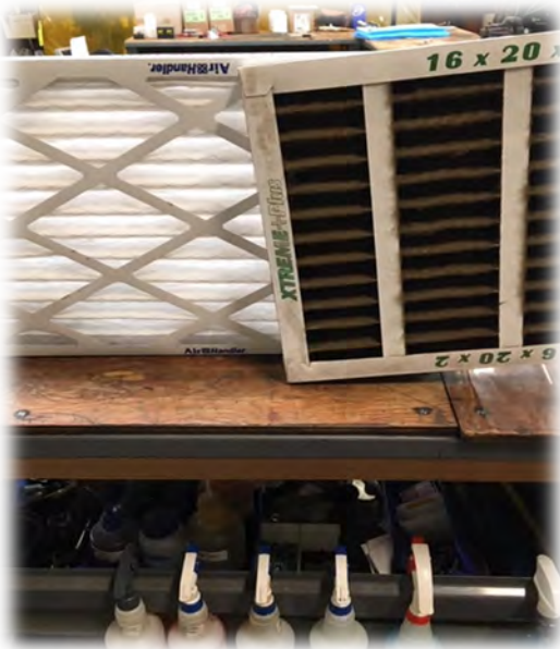
3) HVAC filters new and old
