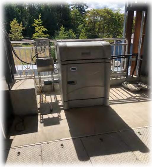
1) New Influent Sampler installed
