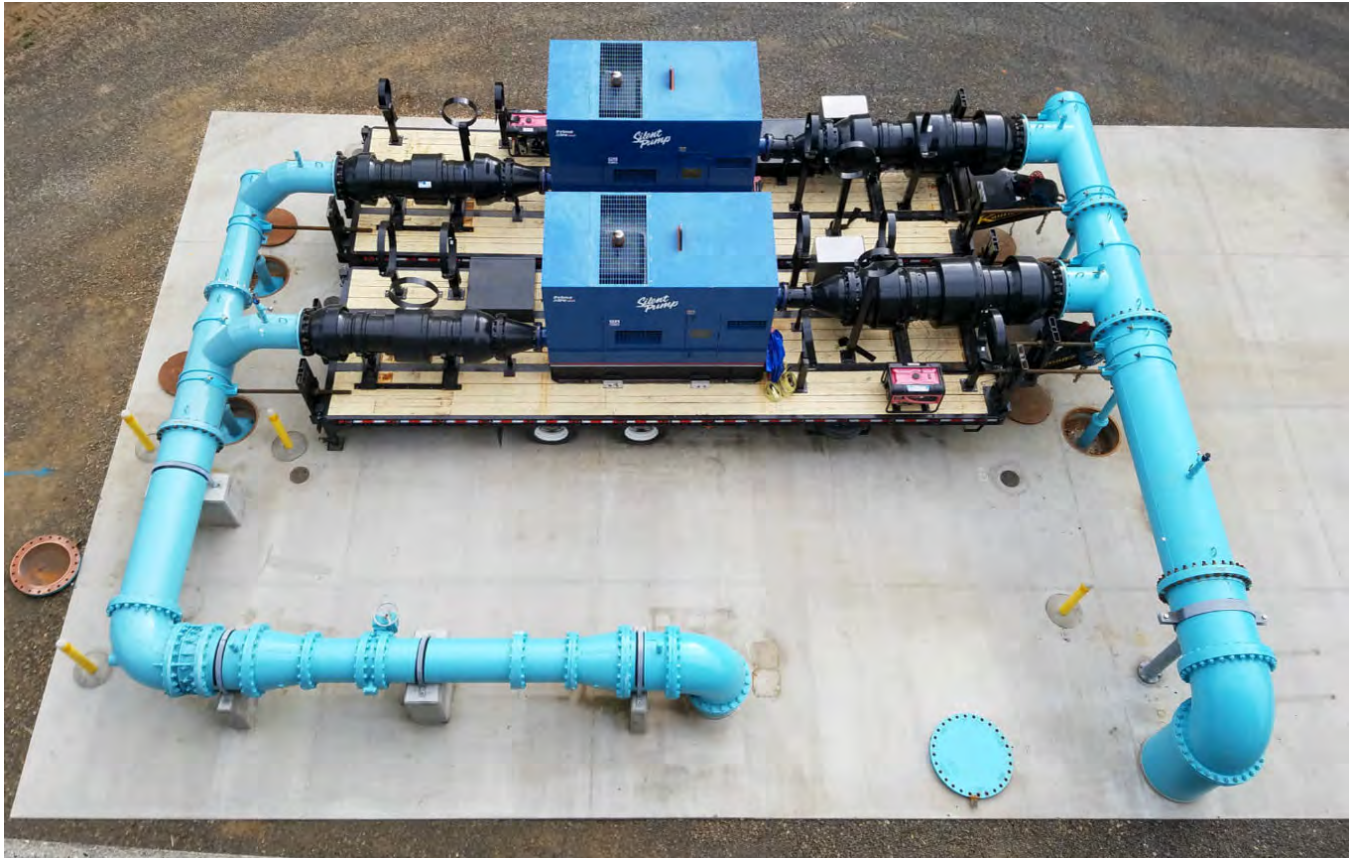
Figure 5-5. Example of Portable Trailer-Mounted Pump Station from TVWD
