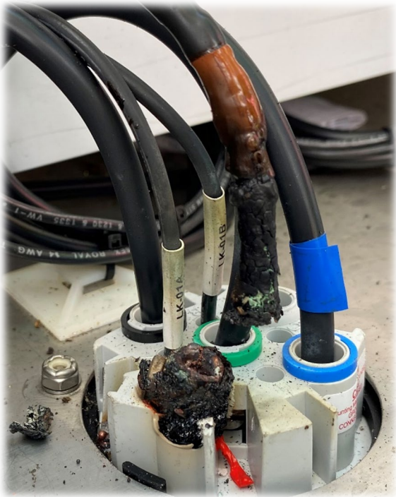
Lift Station #5 severed Power on Pump 1
