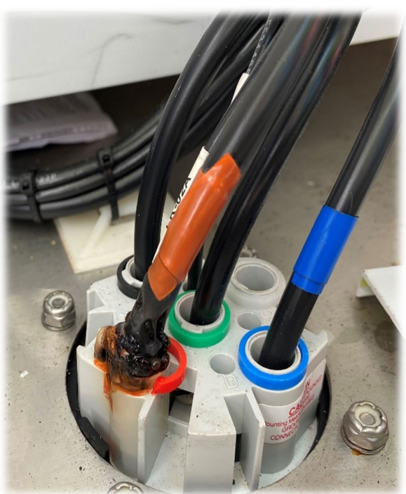
Lift Station #5 Pump 2 wire on the brink of failure
