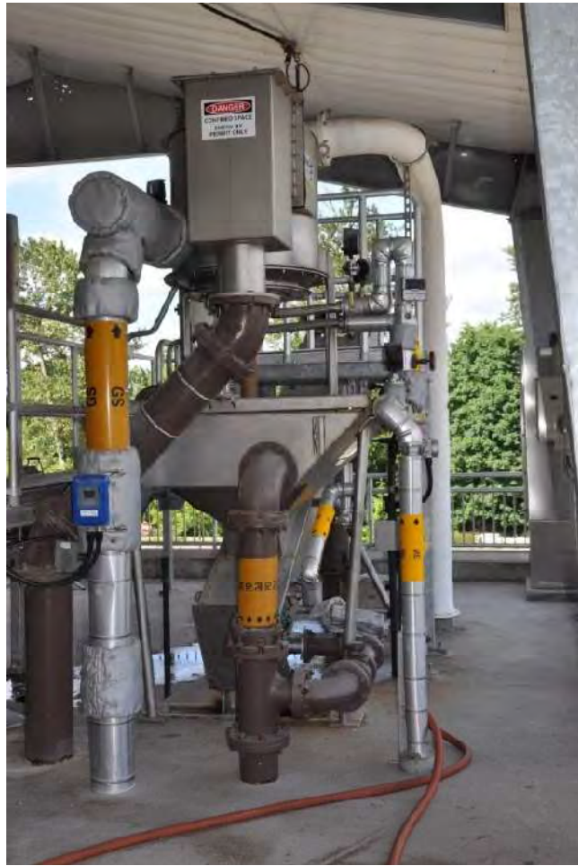
Figure 19. Grit washing and dewatering equipment
