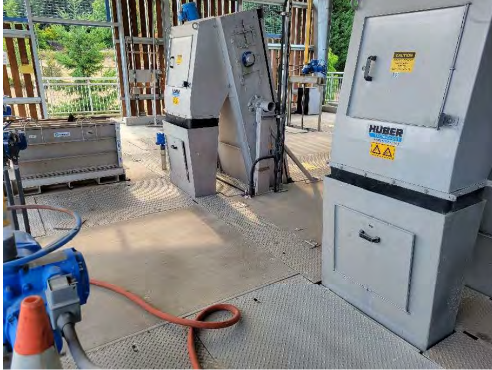
Figure 11. Multi-rake influent screens
