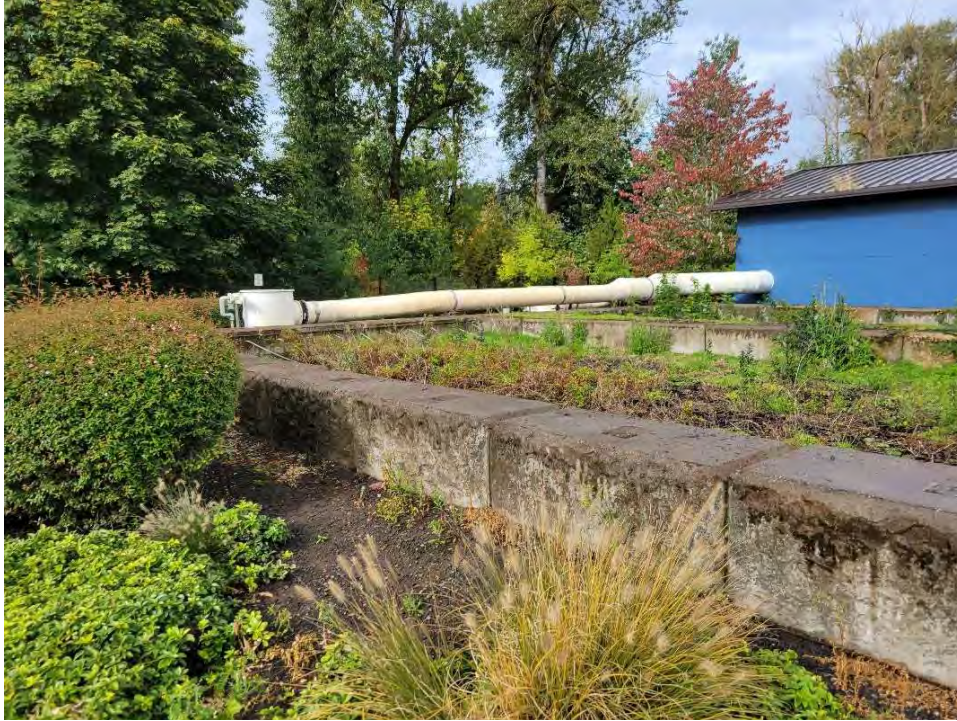
Figure 52. Biofilter building and foul air piping
