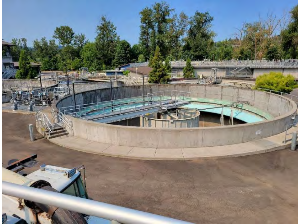
Figure 29. Original secondary clarifier
