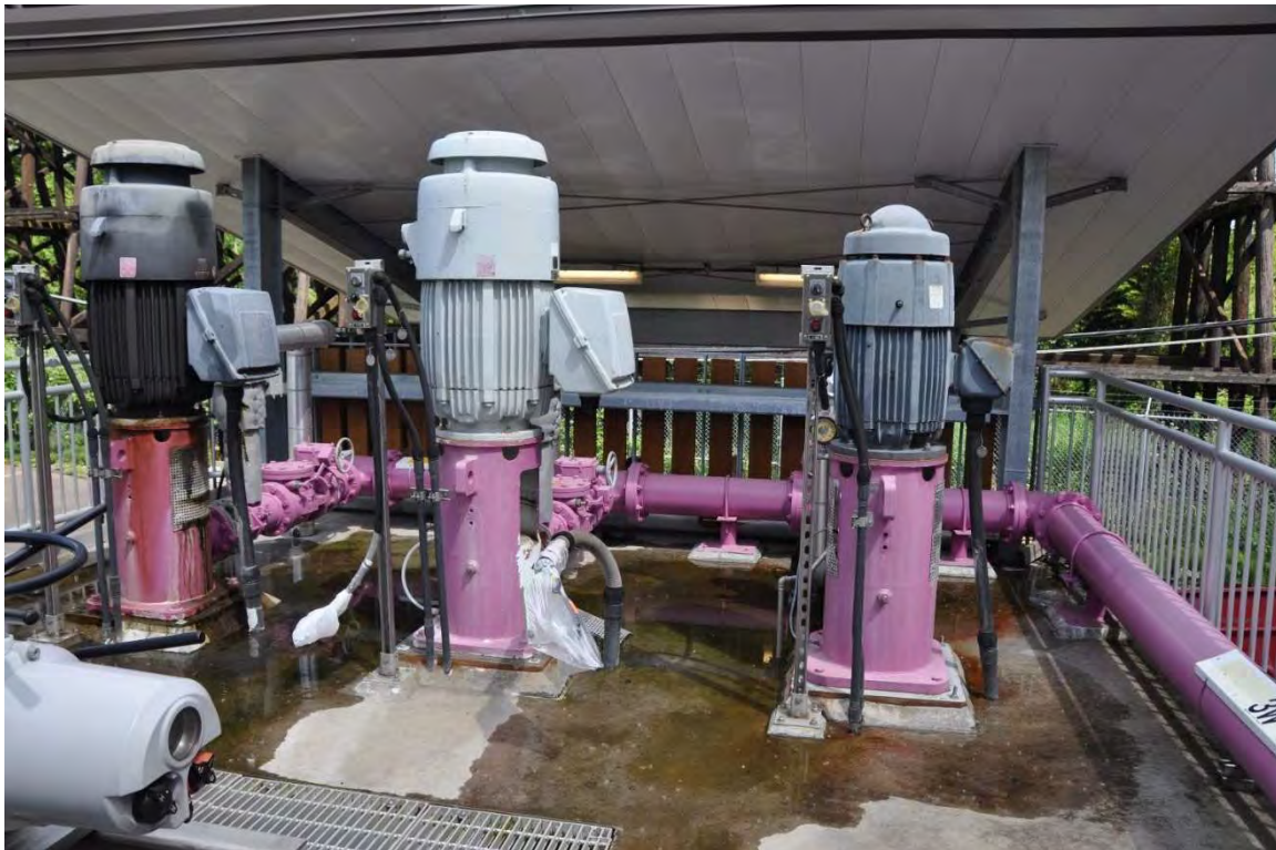
Figure 34. 3W pumps located at the disinfection facility
