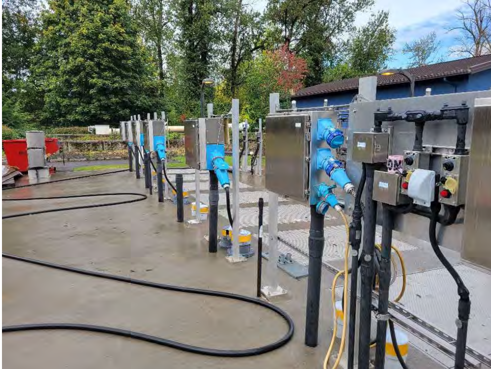
Figure 4. IPS and Plant DPS controls at grade
