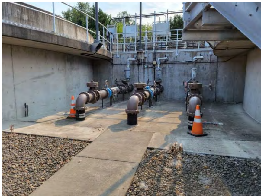
Figure 25. RAS pumps at Secondary Clarifiers 3 and 4
