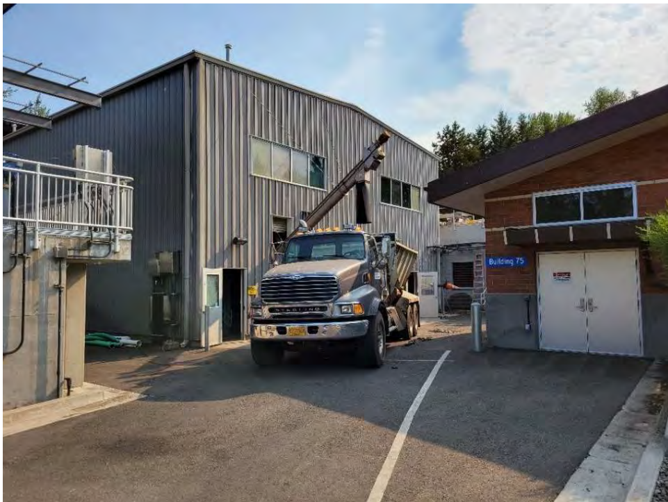
Figure 46. Truck loadout at Solids Handling Building
