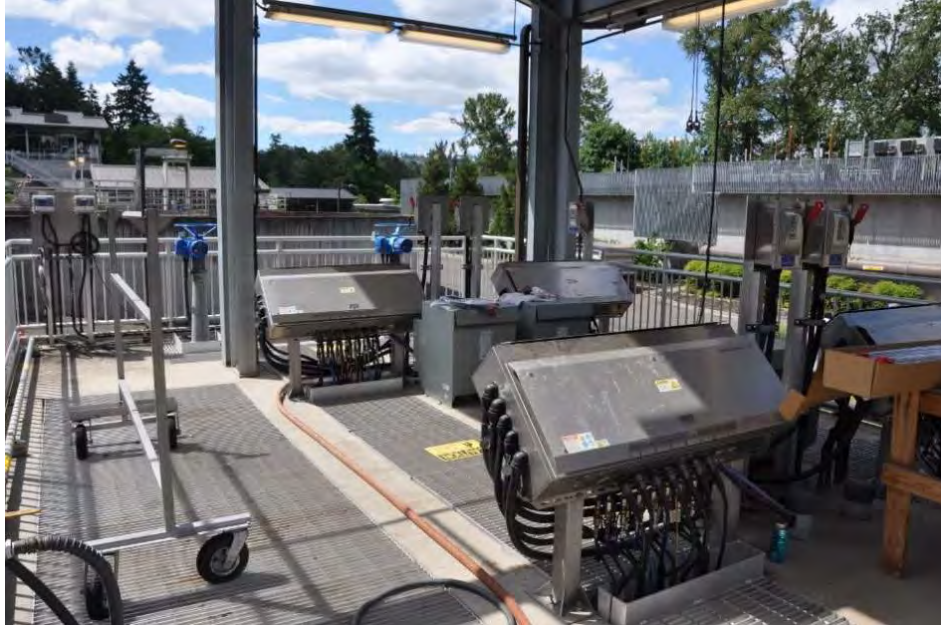
Figure 34. UV channels and equipment
