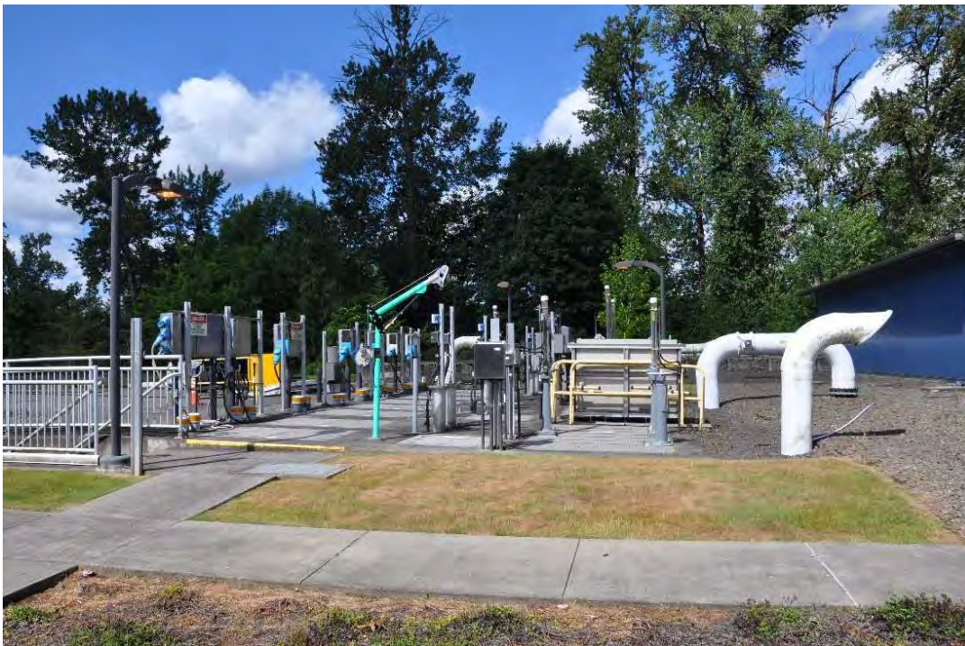
Figure 3. Influent Pump Station and Plant Drain Pump Station at grade
