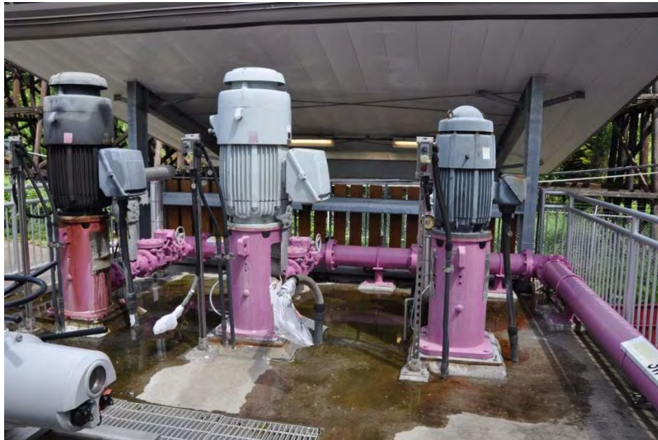
Figure 50. 3W pumps located at disinfection facility
