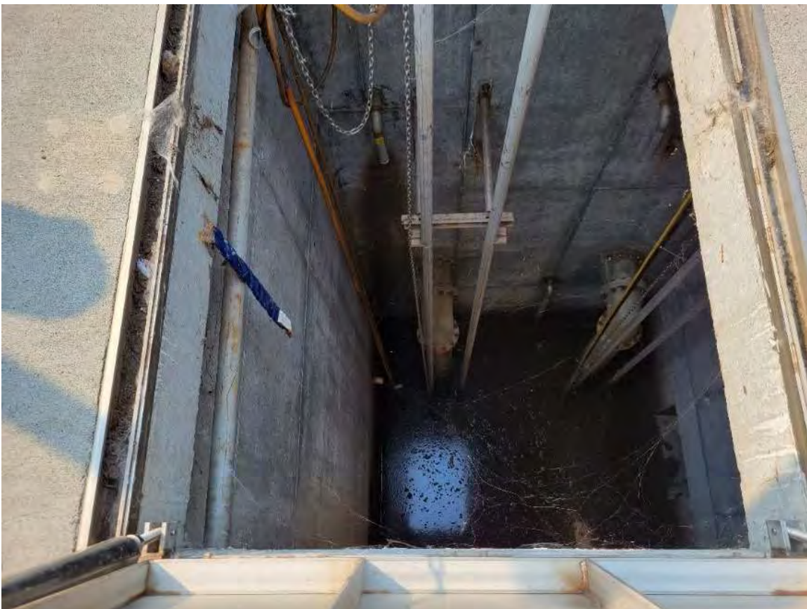
Figure 5. Drain pump station wet well
