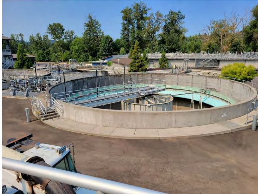
Figure 22. Original secondary clarifier
