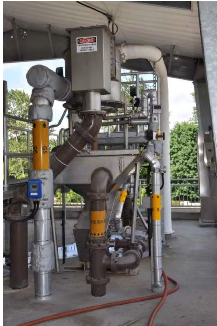
Figure 14. Grit washing and dewatering equipment
