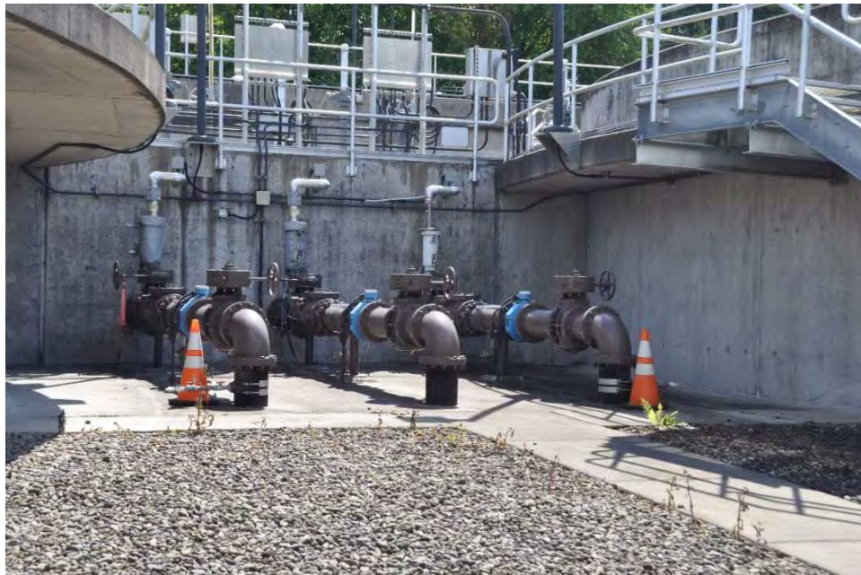
Figure 33. East RAS pump discharge
