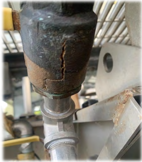
Another Broken pipe due to Freezing.
