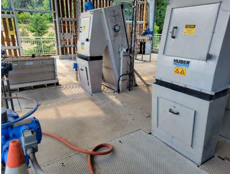
Figure 10. Multi-rake influent screens
