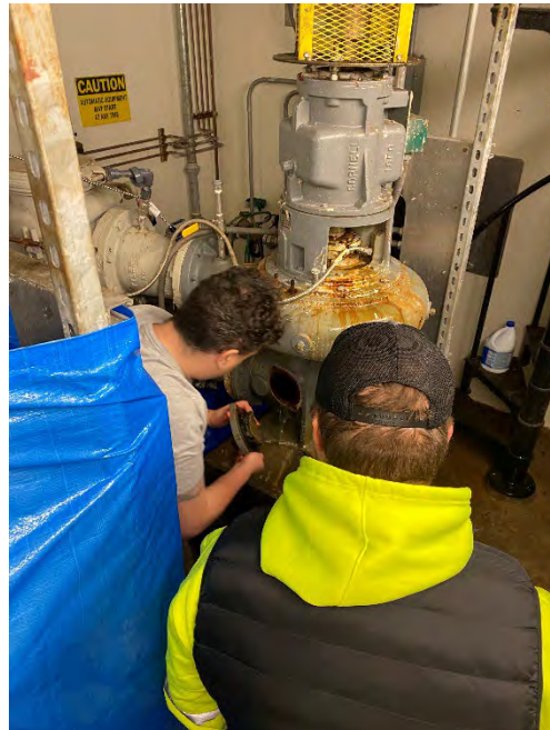
Pump Station Maintenance Training
