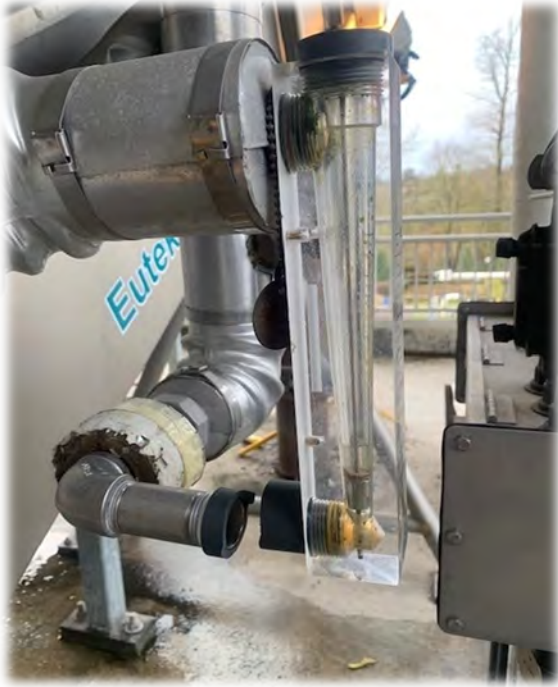
Broken Rotometer due to Freezing.
