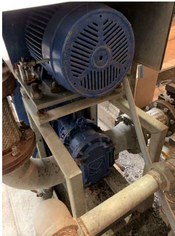
Figure 44. Thickened waste activated sludge pump
