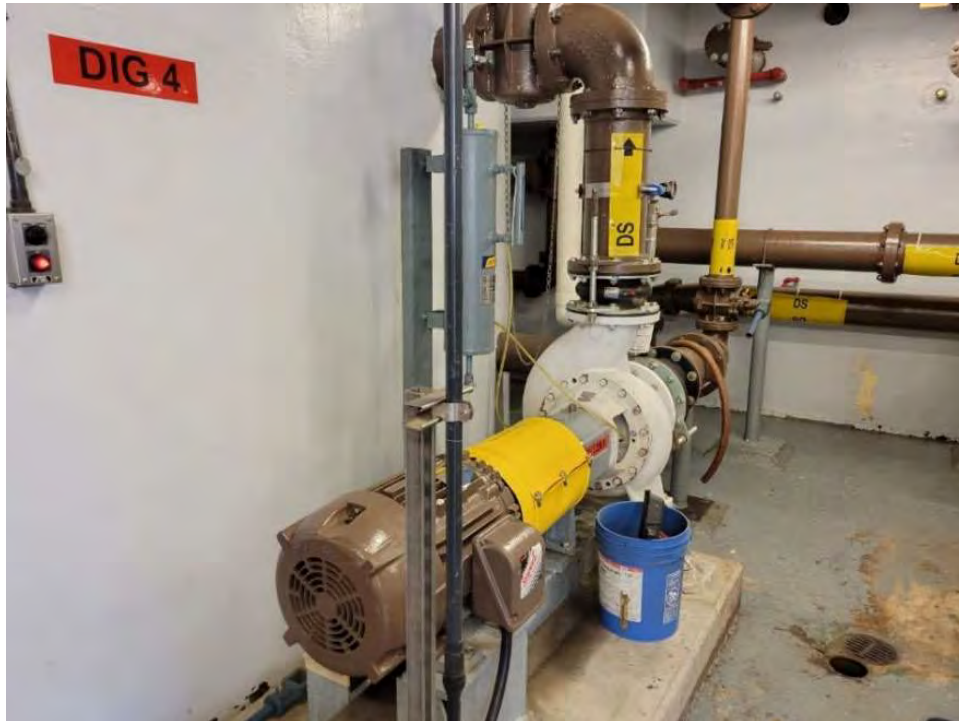
Figure 30. Digester mixing pump
