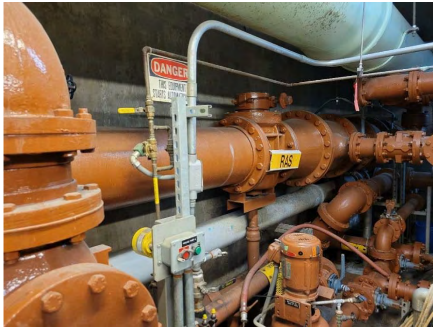
Figure 20. Older WAS pump
