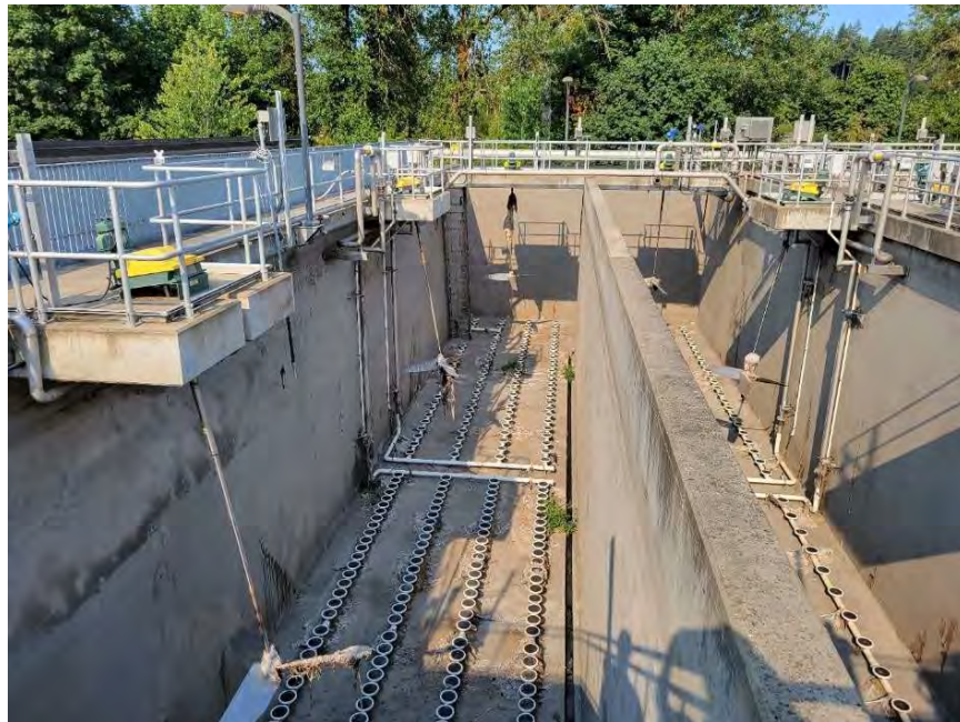
Figure 16. Aeration Basin 1 with mixers visible
