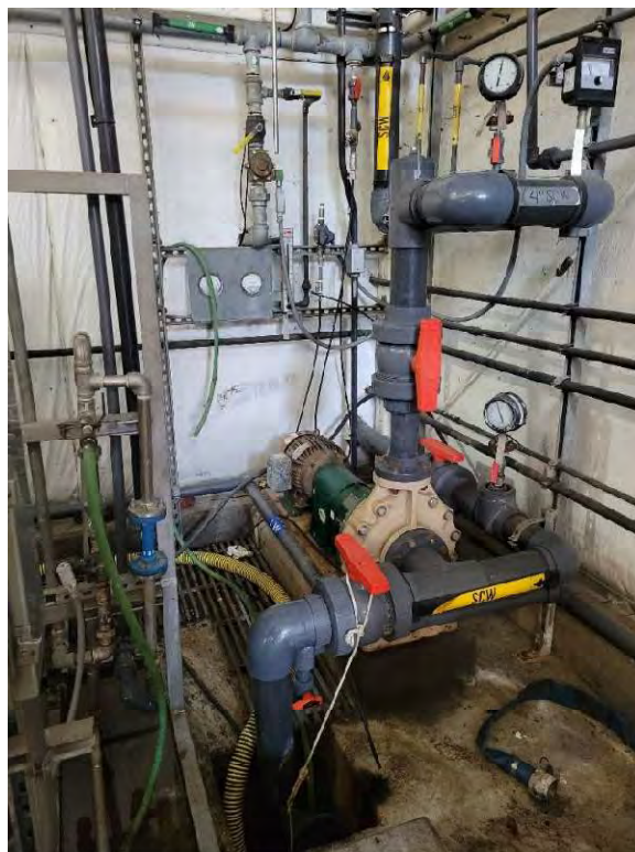
Figure 54. Chemical recirculation pump
