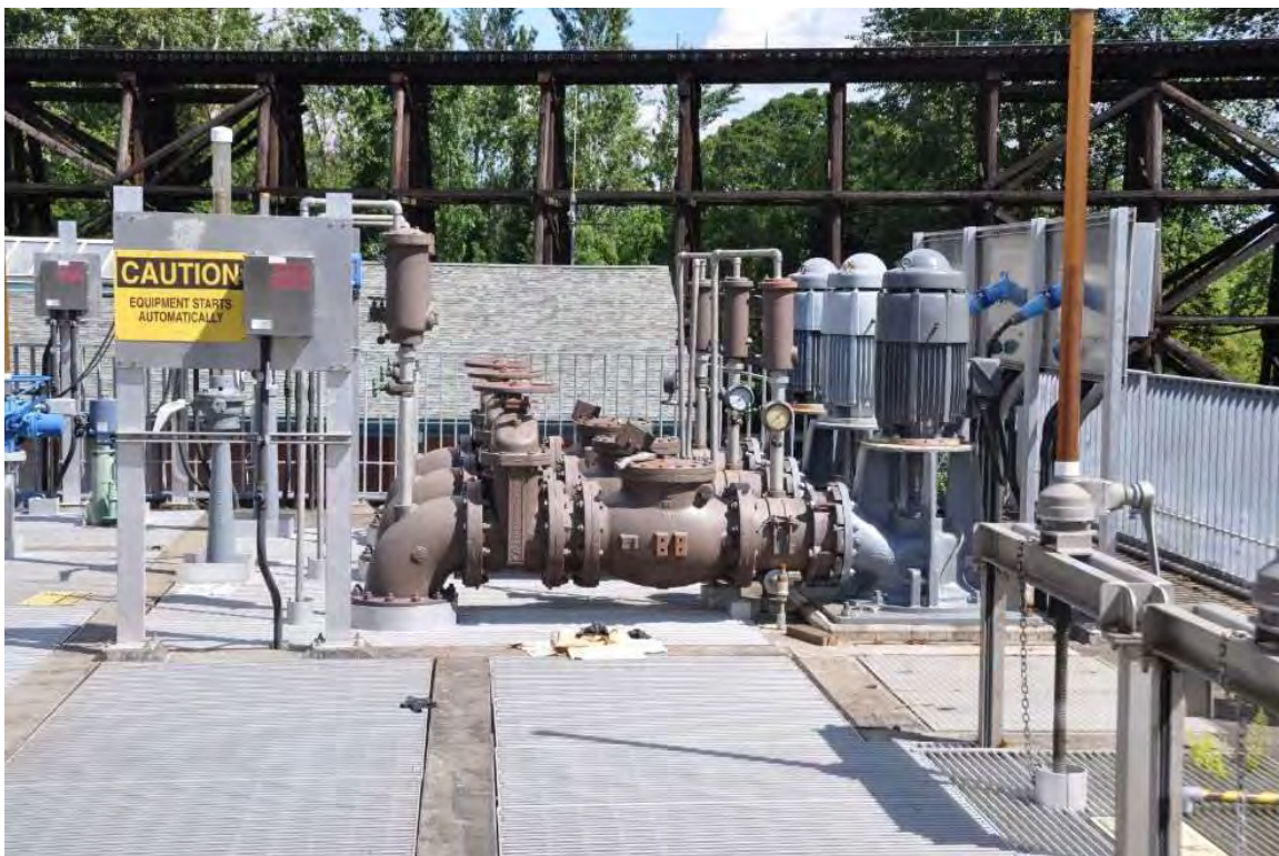
Figure 25. Internal mixed liquor recycle pumps
