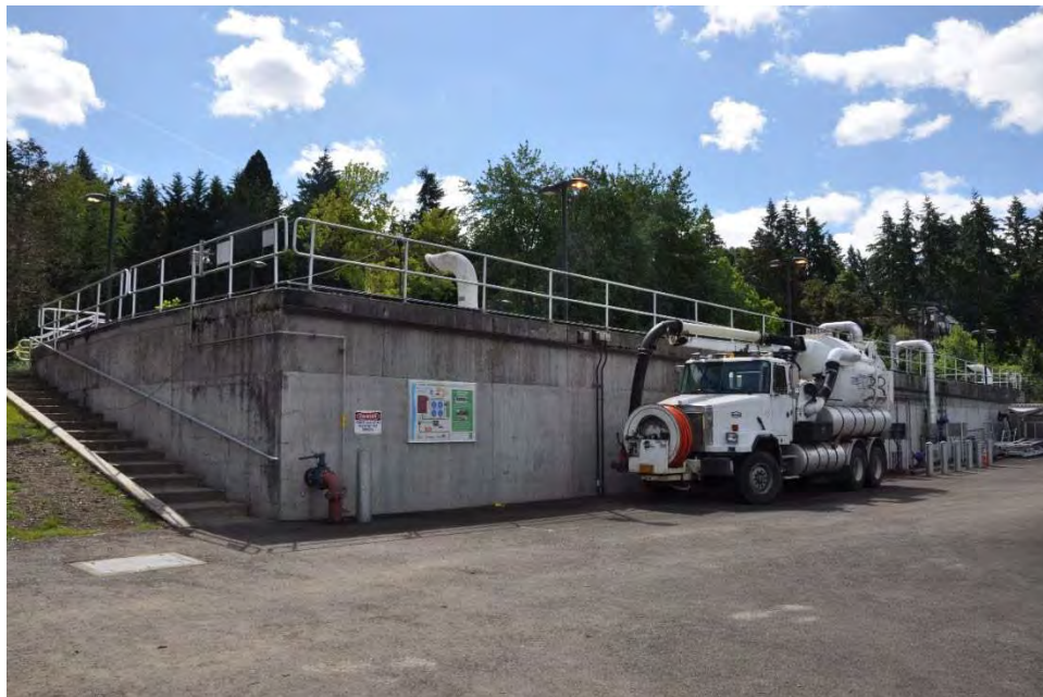
Figure 37. Aerobic Digesters 1 and 2 from below
