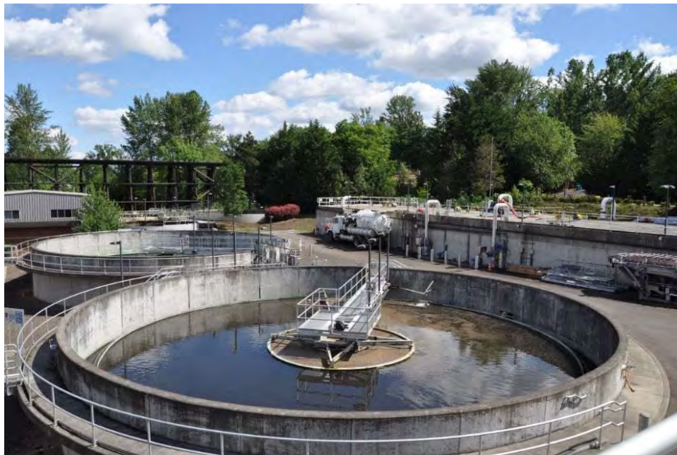
Figure 30. Newer secondary clarifier
