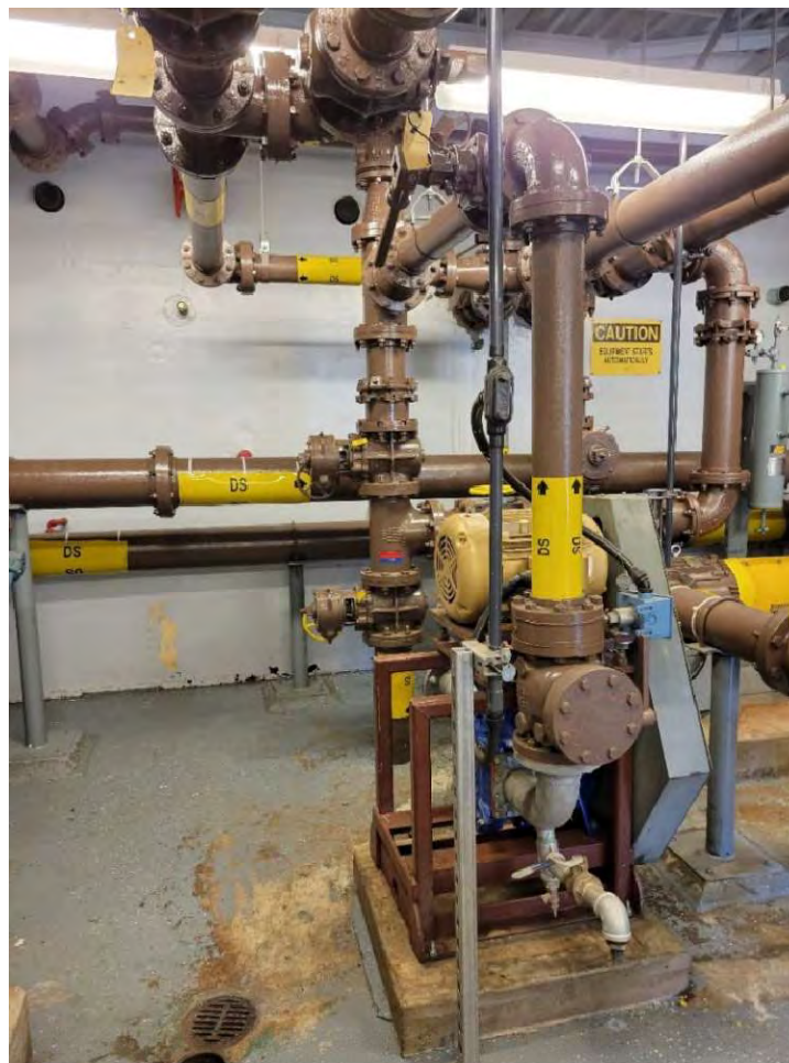
Figure 42. Digested sludge pump
