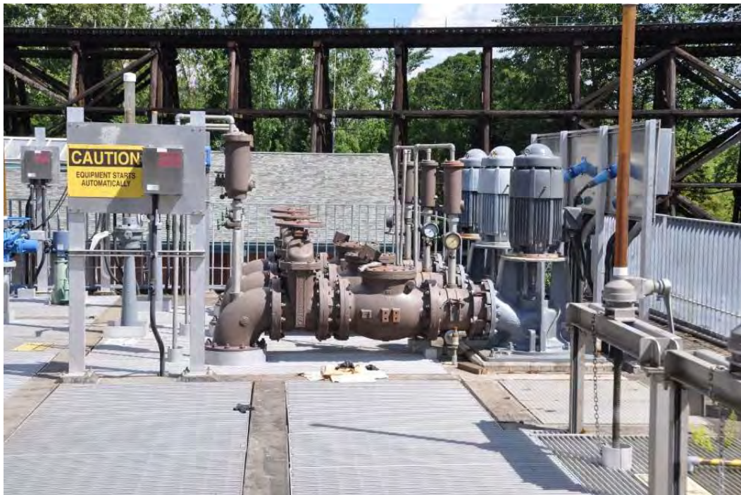
Figure 19. Internal MLR pumps
