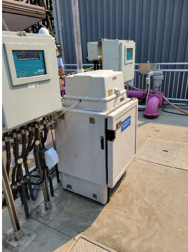
Figure 27. Effluent flow meter panels and composite sampler
