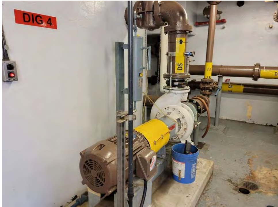
Figure 40. Digester mixing pump
