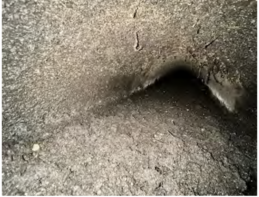
Photo 2: Sediments and debris impacting stormwater piping
