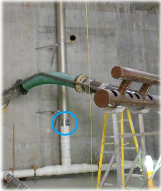
Suspected Bad Clamp in Digester
