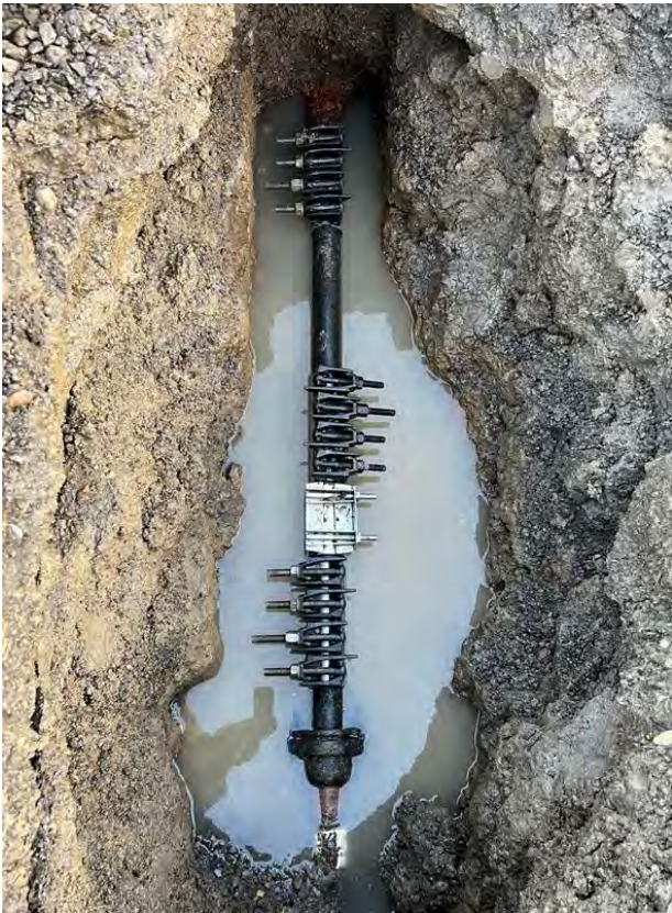
Photo 5: Attempts to fix pipe with clamps
