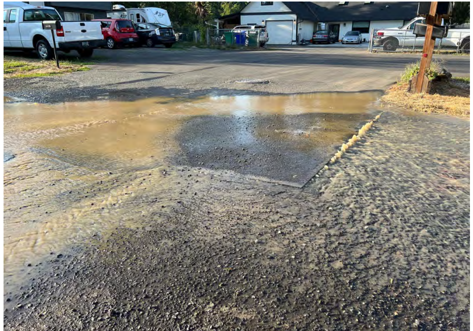
Photo 4: Effects of leaking 2-inch cast iron on Blanton Street
