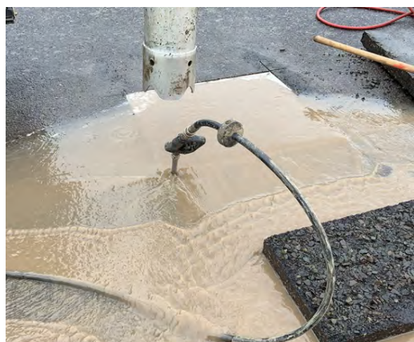
Photo 6: Service leak on Quiet Meadows Rd
