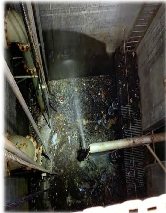
Filthy influent pump station after the excess flows.
