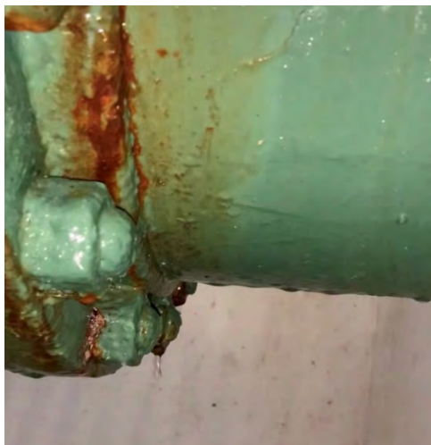
Photo 5: Slow leak in piping at Valley View
