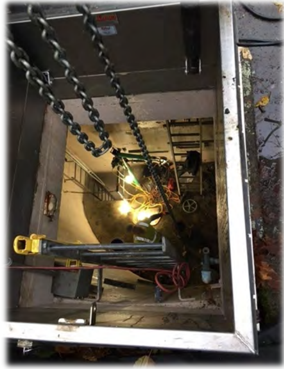
Interior of Lift Station #5.
