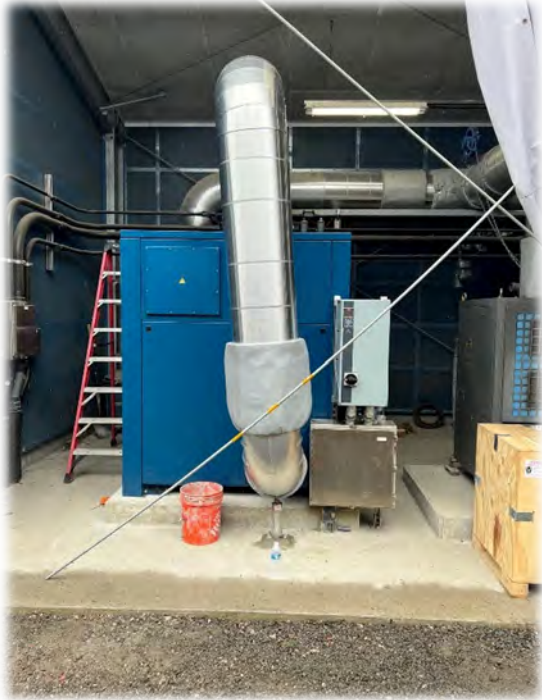
Aeration blower #4 Aerzen Install.
