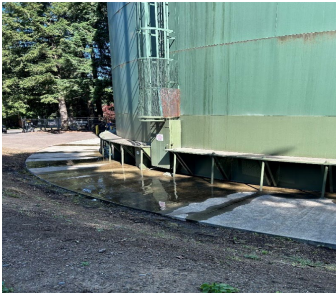
View Acres Reservoir Leak
