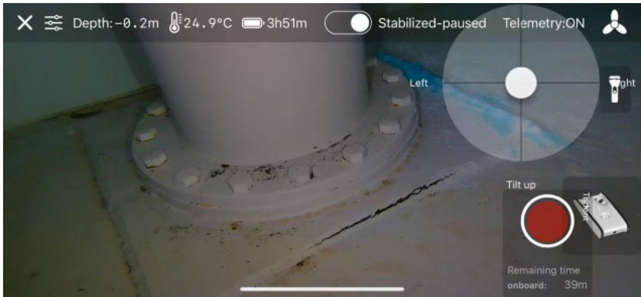
Second Cracked Weld Forming on Inlet Pipe Doubler Plate
