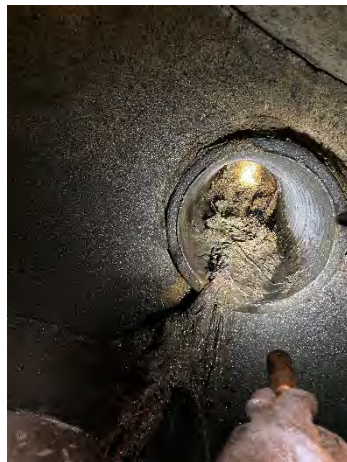
Roots in Storm Line
