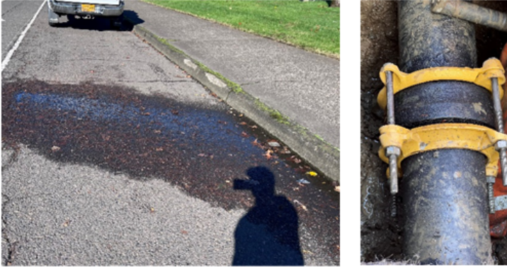
Above - Bell Joint Leak on McLoughlin Blvd. Investigation of leak (left), and repair (right)
